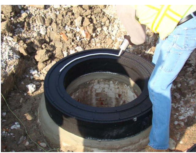
7. If multiple Grade Rings are required, repeat step 6 until all Grade Rings have been properly installed and then proceed to step 8.
